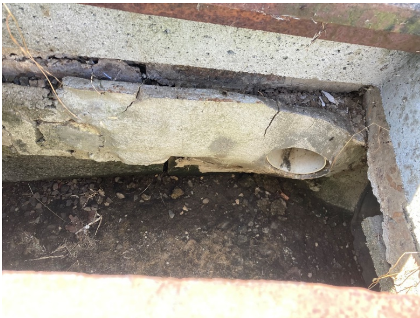
Fig. 3. Catch basin 6394. Homemade catch basin falling apart. Replacement is needed.
