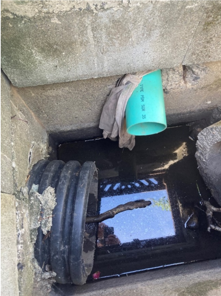
Fig. 1. Catch Basin 6504. All openings need to be grouted and sticks removed.
