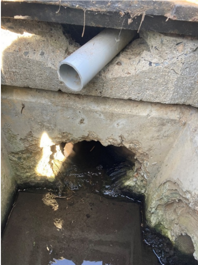
Fig. 2. Catch basin 6505. All penetrations and openings need grout repair.
