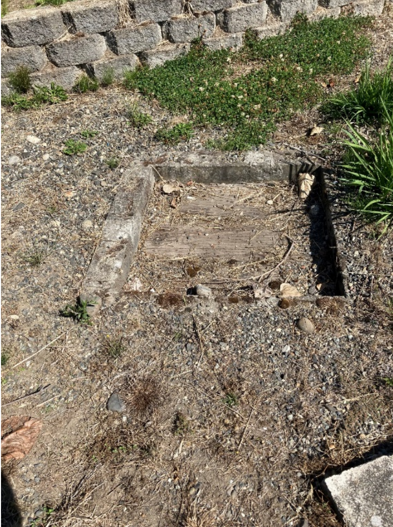
Fig. 4. Catch basin 6392. Several catch basins have no grate or any type of access. These are a safety hazard and need to be repaired in order to perform catch basin inspections.
