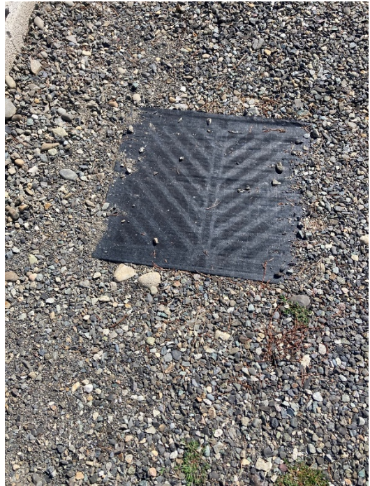
Fig. 10. Catch basin 6376 at 5549 Bay Ridge Drive. The grate is covered with filter fabric. coordinate the home owner to establish an ongoing inspection schedule for CB.
