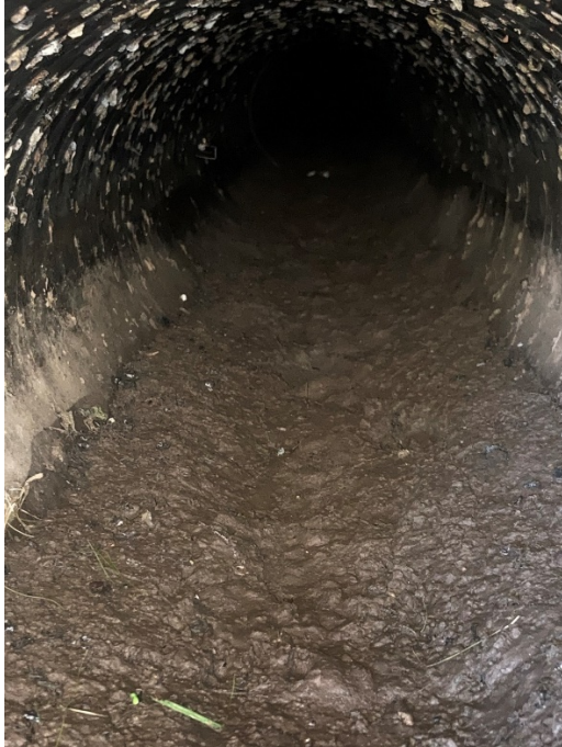
Fig. 9. Storm pipe running along Bay Ridge Drive. Major sediment build-up and jetting is needed.
